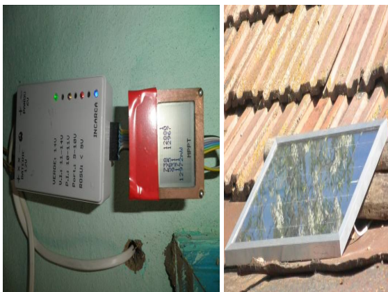
Fig.15. Controller and solar panel under real use.
